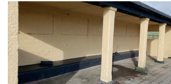
Insufficient protection of built heritage
